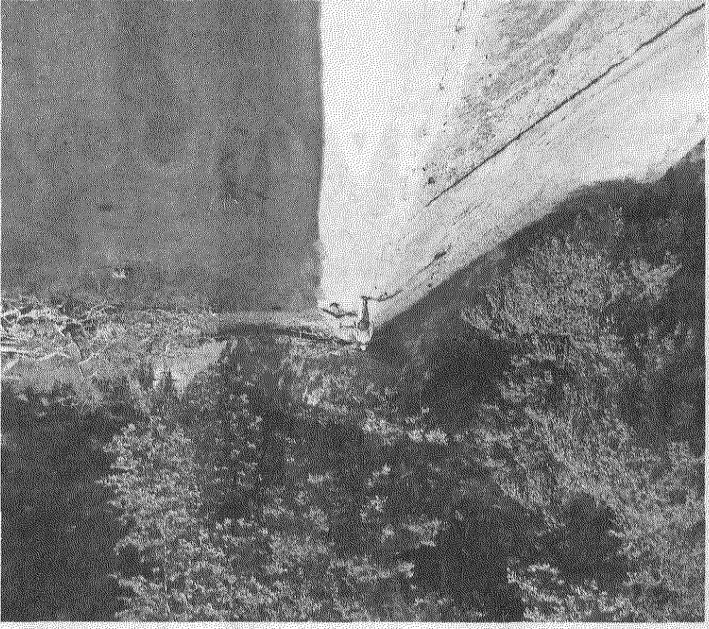
The Warren Glen Dam on the Musconcong River between the Warren Glen section of Pohatcong Township and the Bloomsbury area is seen in 2016. A person standing on the dam gives a sense of scale. Courtesy of Musconcong Watershed Association
