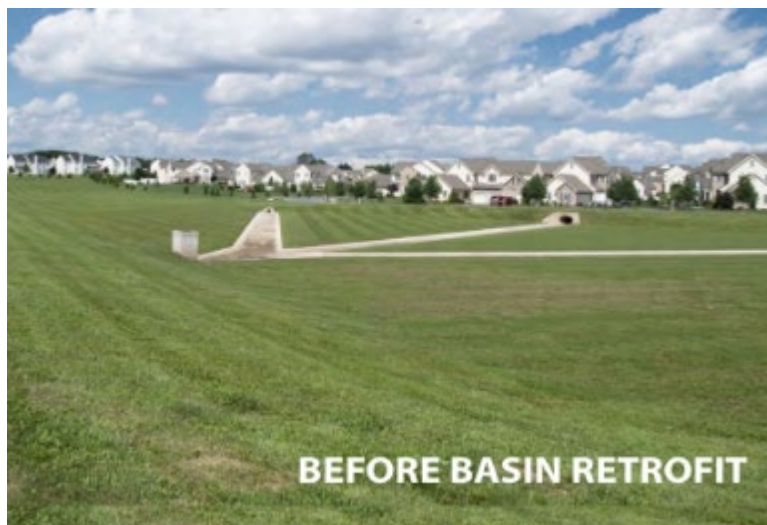
Figure P.7 – Low flow concrete channels directing all stormwater to one area. Turf grasses shallow roots are not able to soak up much water or create channels in the soil for water to infiltrate.
