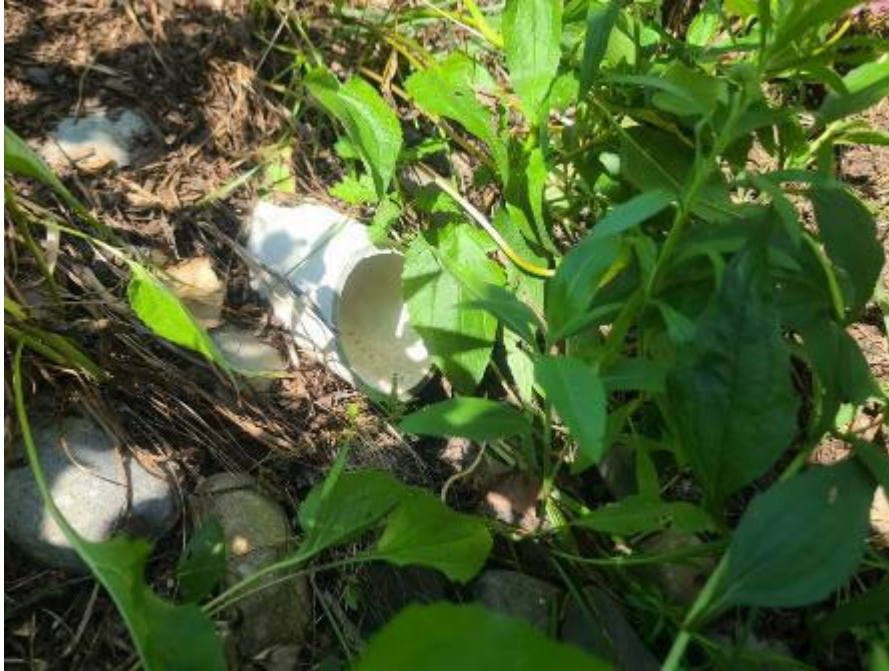
Figure P.3 – End of pipe into Rain Garden bed. Photo credit - MWA
